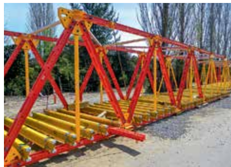
In order to ensure accessibility, the horizontal bracing is mounted on the outside of the pedestrian bridge by means of a simple, clever solution.
