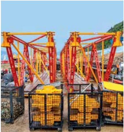
Pre-assembled girder packages can be temporarily stored on site using only a minimum of space until they are lifted to the next place of use.
