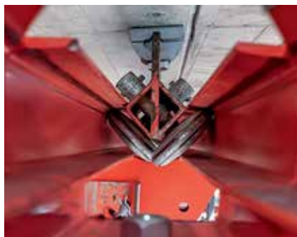
The VARIOKIT Cantilevered Parapet Track was suspended by means of rails and Roller Units from the underside of the bridge cantilever – at an identical position to the moving procedure and concreting.
