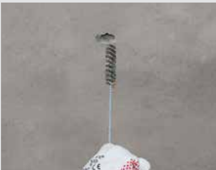
Step 1 Drill hole with d = 22 mm and t = 160 mm (at right angles to the concrete surface); cleaning the drilled hole with brush and blow-out pump
